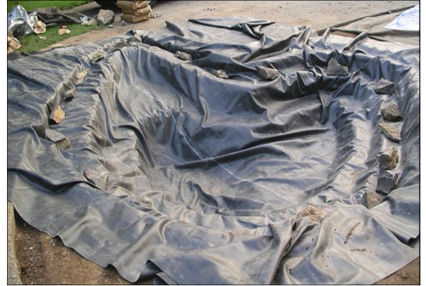
A pond liner installed showing shelves in the pond for different types of plants.
